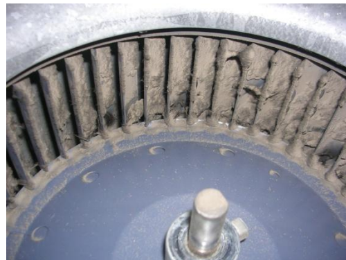
Dirty blower wheels decrease efficiency and increase repair costs.
